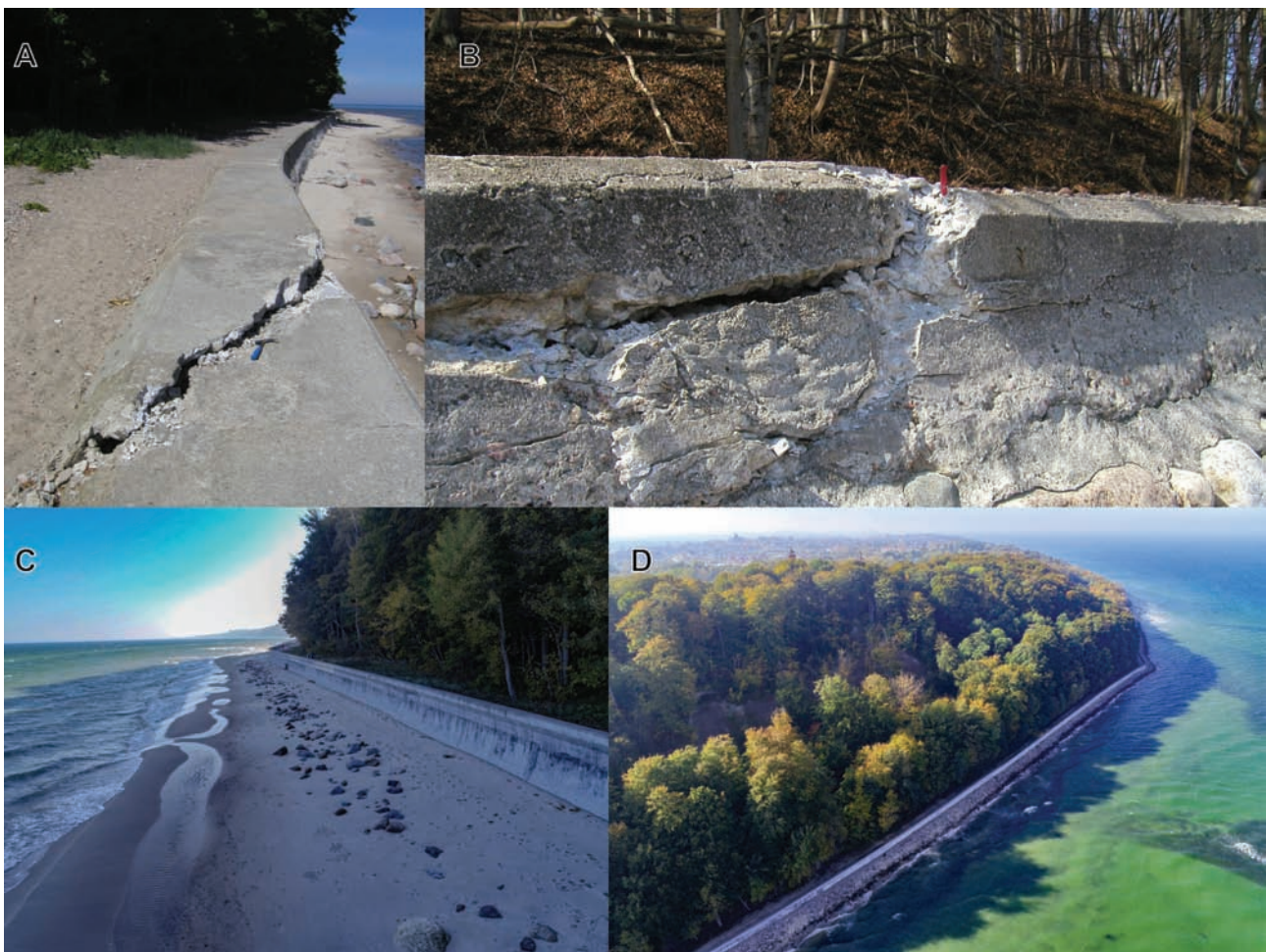
Fig. 2 Damaged (A, B – photo: L. Jurys) and the rebuild and expanded (C, D – photo: M. Olkowicz) seawall at Rozewie headland
